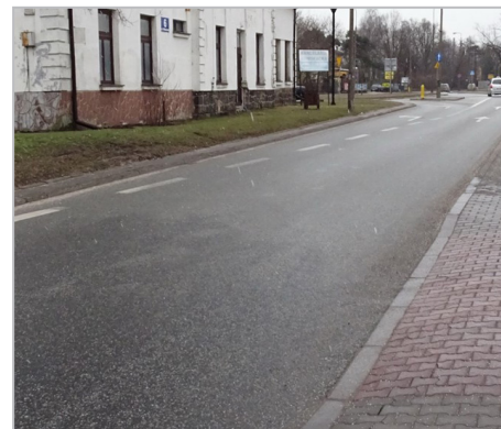
February 2016 — Inspection after 10 years. Nearly 10 years later and still no signs of damage to the wearing course.
