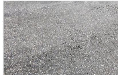
Condition in 2020 — first signs of deterioration after nine years; damage is not considered significant enough for the road to be repaired yet
