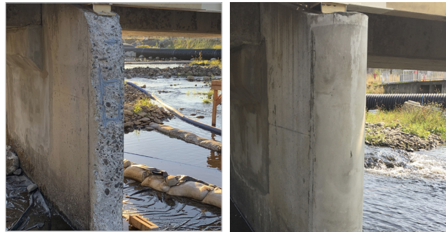
The contractor fabricated custom forms to enable access to the repair area for application of the RPS-752 bonding agent and speedy pour of RPS-263 rapid-hardening repair mortar.
