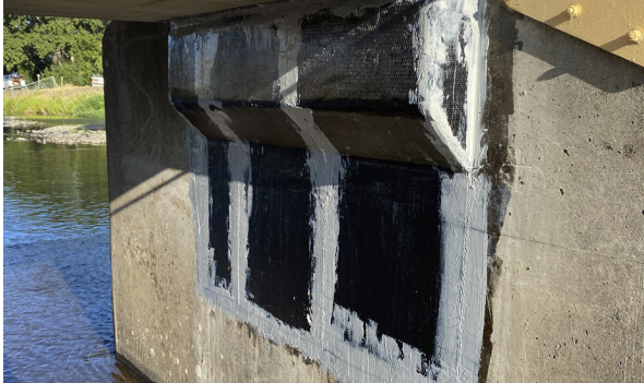
CSS-CUCF11 carbon FRP was installed over the repaired corbel to extend the life of the structure and assist in preventing future deterioration.
