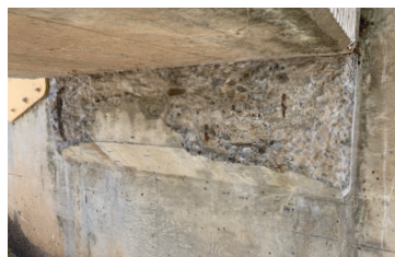
The corbel was deteriorated beyond what was expected, creating significantly more repair work prior to FRP installation.
