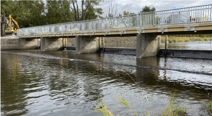
Completed project with damaged sections repaired, strengthened, protected and seamlessly blending with the original design.
