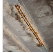
Exposed rebar prior to repair of the risers.
