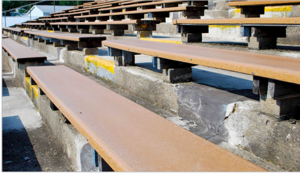
The top of the grandstand area prior to repair.
