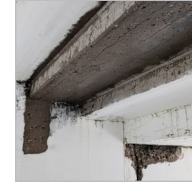
Cracked riser showing water leakage and cracking which needed to be repaired. Paint was removed prior to repair.
