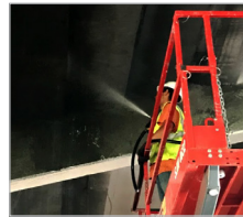
Sprayability made FRCM an attractive option as a repair mortar for overhead installations.
