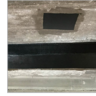
The mezzanine area was hand-patched with trowelable repair mortar, then strengthened with FRP.
