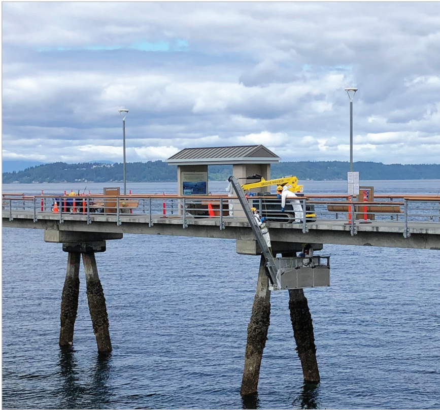
Installation of FRP using the Bridgewalker under-bridge access machine in place of costlier traditional scaffolding.
