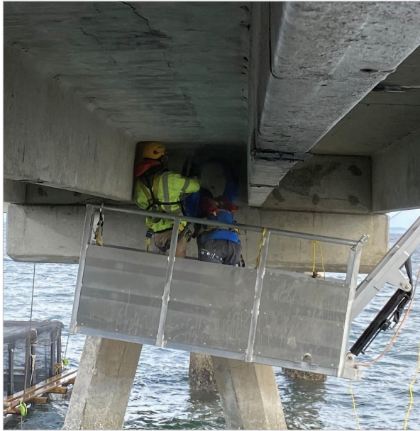
After completion of initial concrete repair, the entire surface needed to be ground to remove contaminants due to saltwater exposure prior to FRP installation.
