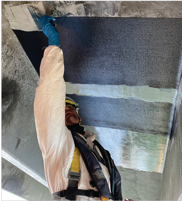
The FRP panels provided structural reinforcement, sealed the underside of the pier against moisture ingress, and eliminated the need to demolish the deficient joint repairs.
