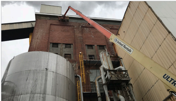
Installation of Heli-Tie™ ties required using a lift to reach heights of almost 120'
