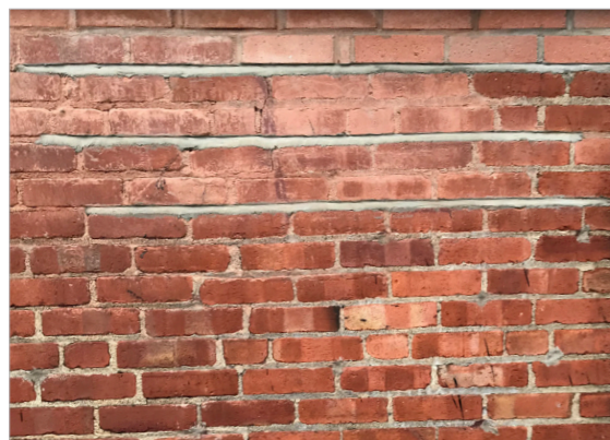
Repointed mortar on the face of the URM wall at Heli-Tie installation locations.
