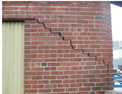
Unreinforced, multiwythe brick wall displayed significant cracking in need of repair.
