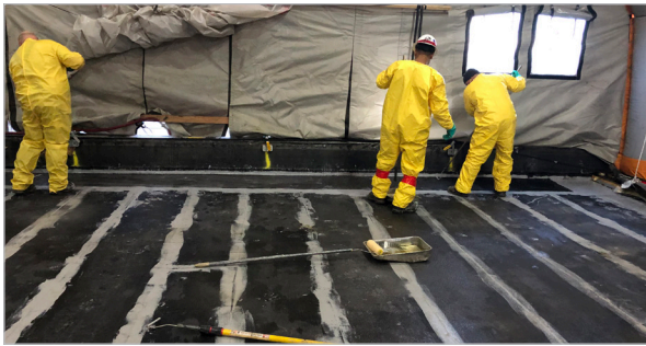
Workers applying a second, perpendicular, layer of in-plane diaphragm reinforcement over the initial layer.
