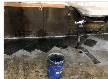
Alternating FRP strips at 45° angles for shear transfer between slab and perimeter beam or wall.
