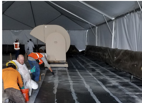
Workers installing FRP strips as in-plane shear reinforcement to the concrete roof diaphragm.
