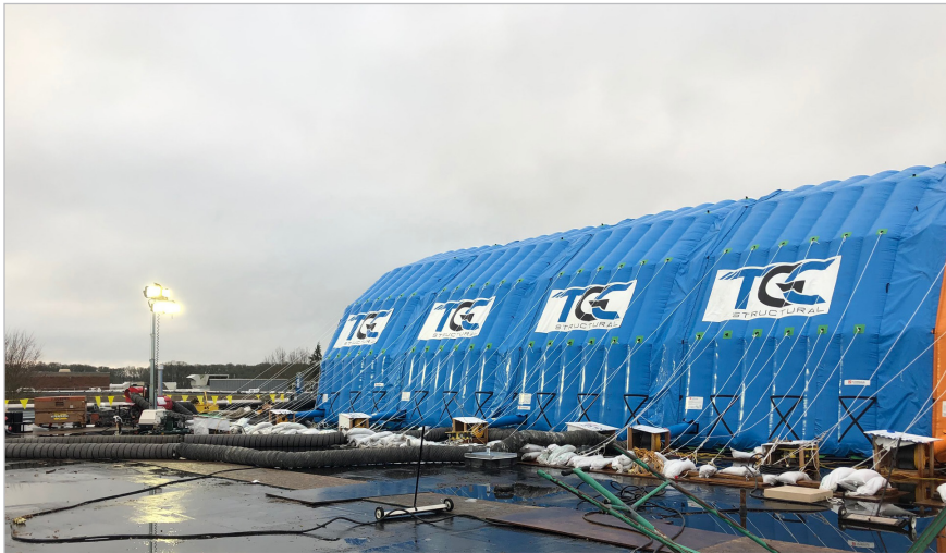
Exterior view of the tenting required to install the FRP at proper temperatures in winter conditions.
