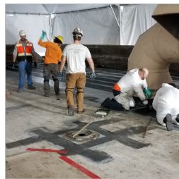
FRP installed around a slab penetration to transfer loads around the opening.
