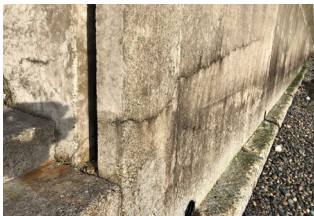
Openings like this allowed for erosion in and behind the wall.
