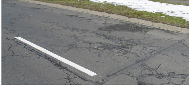
Degradation before repair.
