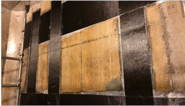
View of completed FRP reinforcement at the interior of pontoons prior to coring for future tensioning cables.
