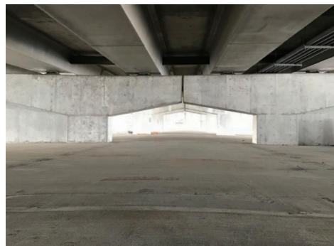
View from on top of the floating pontoon structure and below the bridge deck showing the east-bound I-90 span running adjacent.
