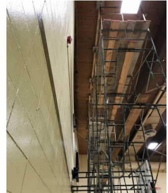
Plane deflection of the wall at the roofline, showing how critical the damage was.
