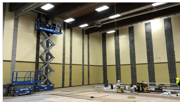
Interior view of FRP installation in progress, showing the vertical strips and spacing needed to retrofit the gym.
