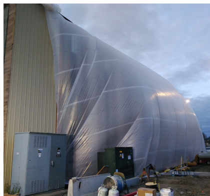
A heated tent was created on the exterior of the gym for FRP installation in Alaska in November.
